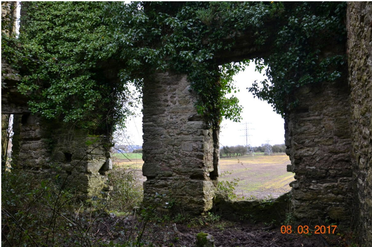
Photo 59 – Area 5. Heavy vegetation, but opes appear to be intact.
