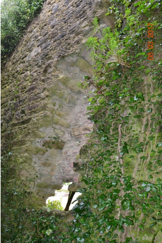
Photo 42 – Area 3. Chimney cuts up through the wall.
