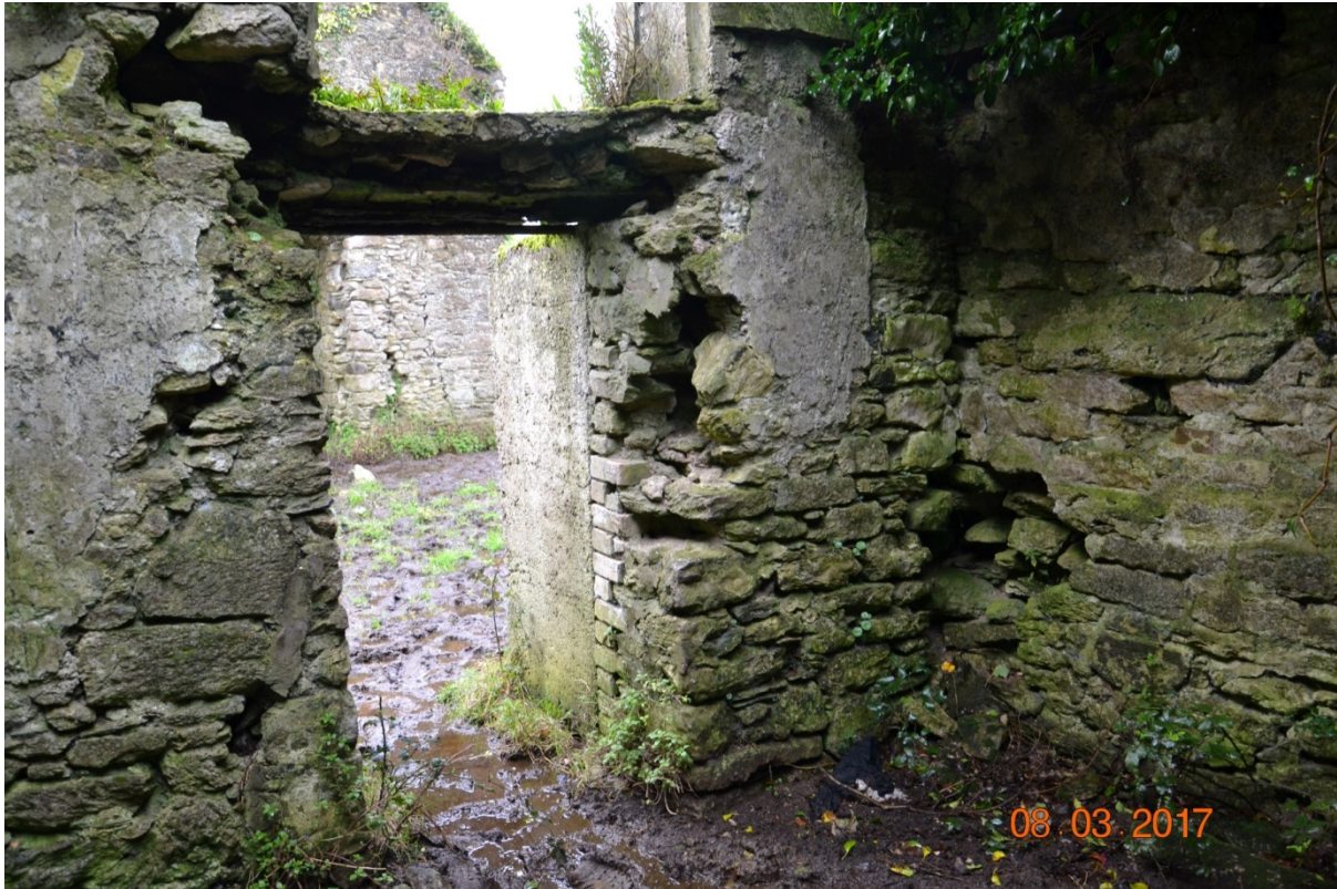
Photo 36 – Area 1. View of missing masonry and deteriorating door lintel.
