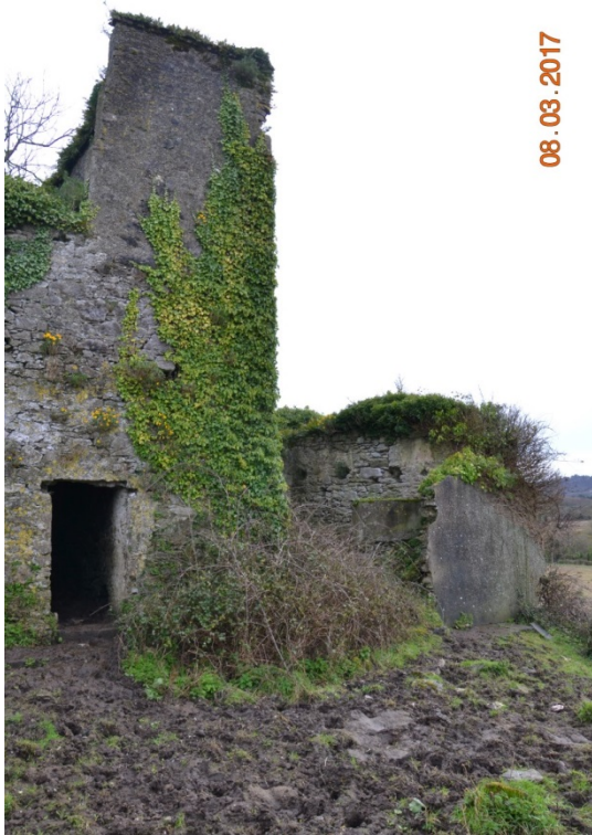
Photo 21 – View of the western elevation of the original structure on the south side.
