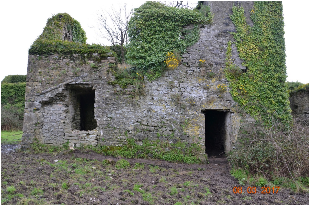
Photo 22 – View of the western elevation of the original structure on the south side.
