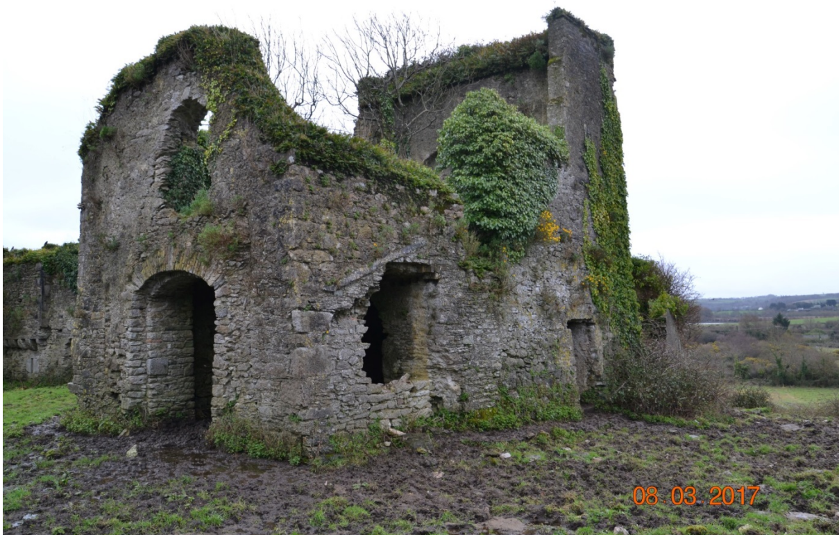
Photo 24 – View of the western & northern elevation of the original structure on the south side.
