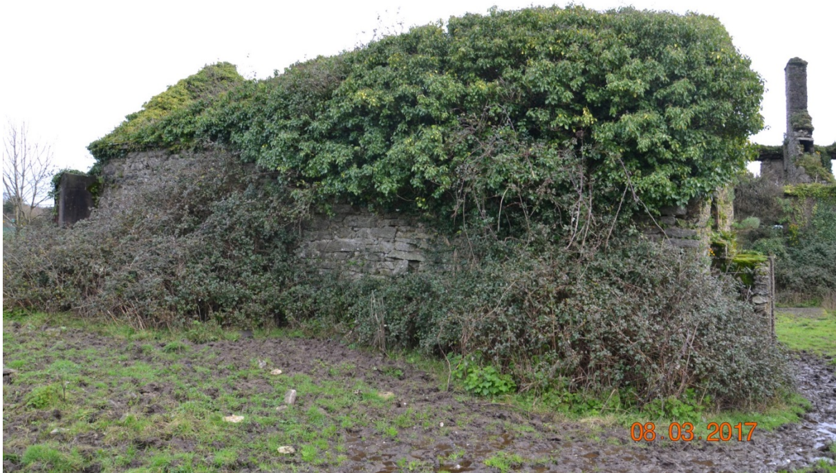
Photo 35 – View of the structure to the north of the entrance to the courtyard. Photo from the West.
