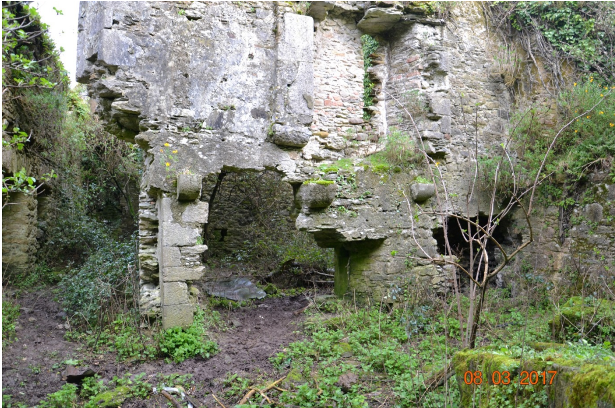
Photo 50 – Area 4. Very significant structural deterioration of the wall between Area 4 and Area 5. Note the stone corbels for supporting the suspended floor beams. The level suggests that the ground level has risen substantially over time.
