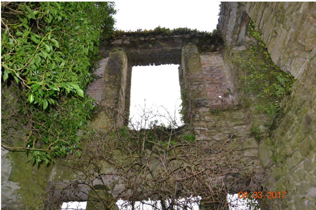
Photo 61 – Area 6. View of the upper ope. Lintel appears to be intact, but looks very shallow / flat.
