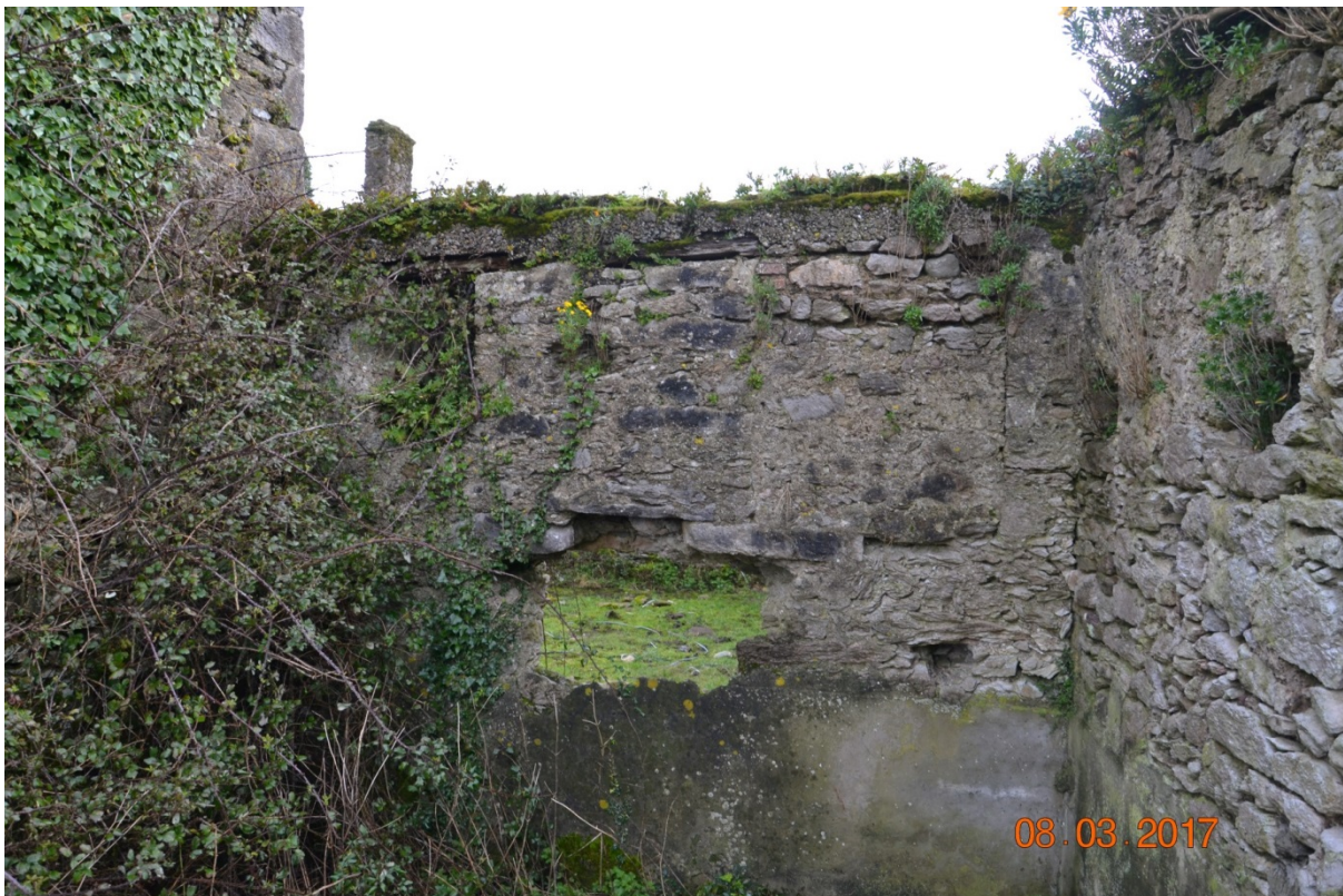
Photo 63 – Area 7. Western elevation of the eastern wall. Note the ope, and the apparent concrete wall capping.
