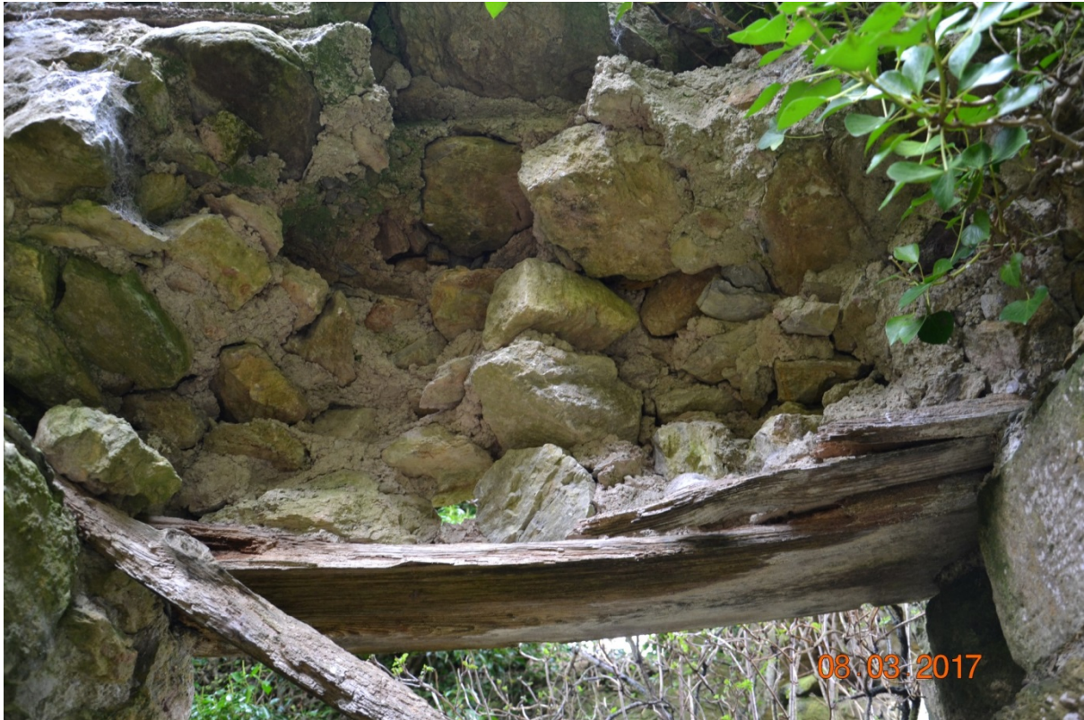
Photo 54 – Area 5. View of the lower lintel – showing significant deterioration.
