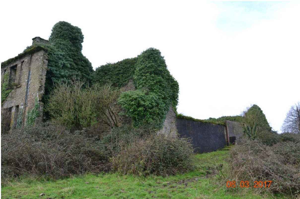
Photo 5 – View of Castle Warren House form the NE – note the vegetation growth.
