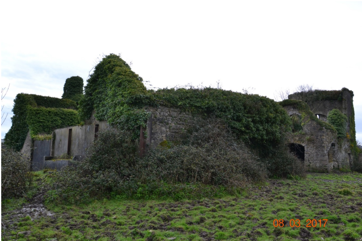
Photo 1 – View of the western elevation of the original structure from the NW – note the vegetation growth.
