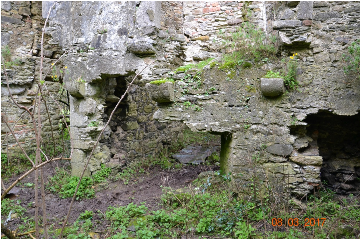
Photo 49 – Area 4. Very significant structural deterioration of the wall between Area 4 and Area 5.
