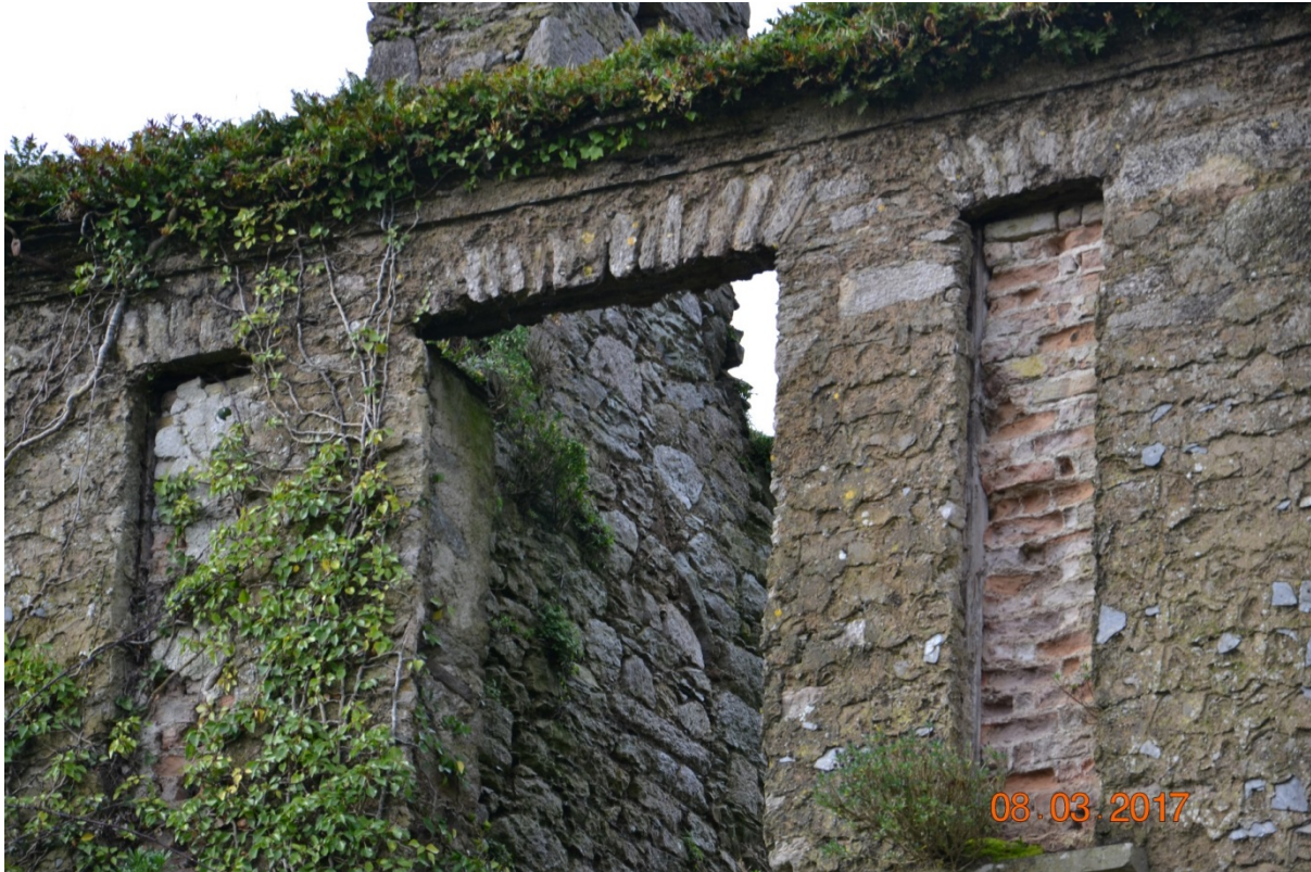
Photo 9 – General view of the lintels over the 1 st floor windows – appear to be intact.
