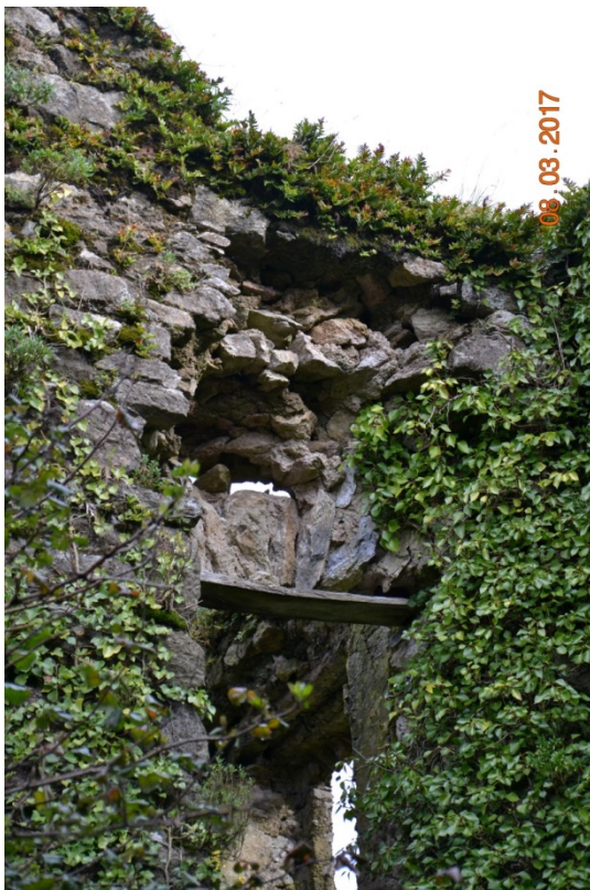
Photo 53 – Area 5. View of the upper lintel showing significant deterioration.
