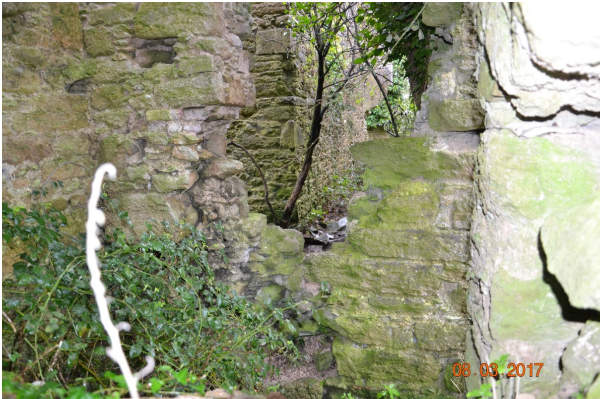
Photo 45 – Area 3. Cill of ope has also deteriorated.
