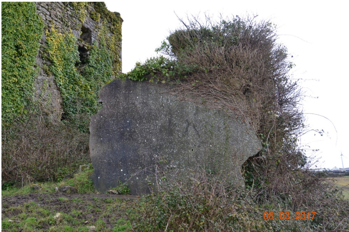
Photo 18 – Concrete wall on the western elevation (South end). Photo from the west.
