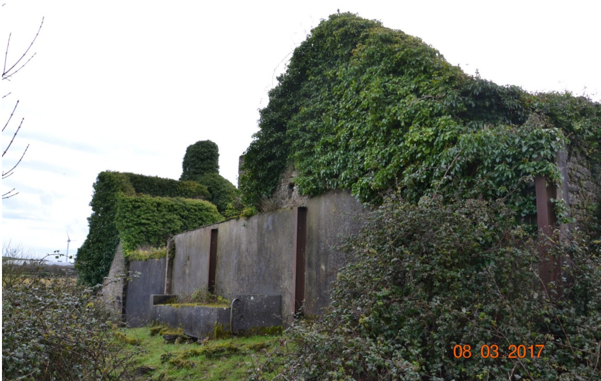
Photo 2 – View of the northern elevation from the NW – note the concrete wall / steel posts.
