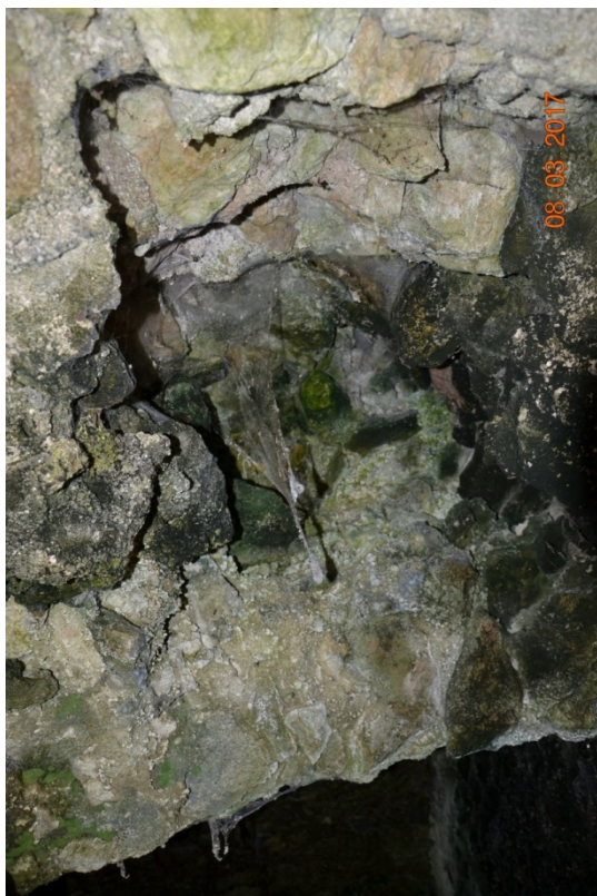
Photo 64 – Area 8. Lintel over the entrance door – shows significant signs of deterioration.
