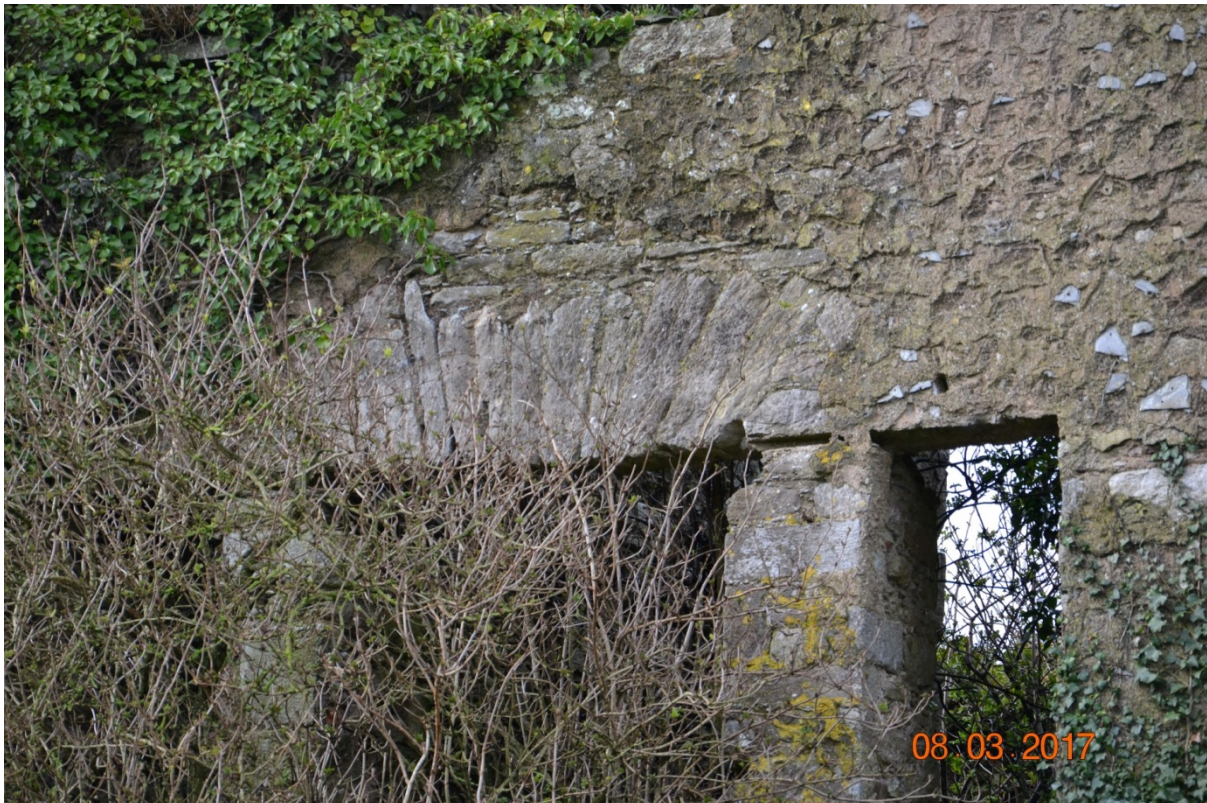
Photo 10 – View of the lintel over the door – appears to be intact.
