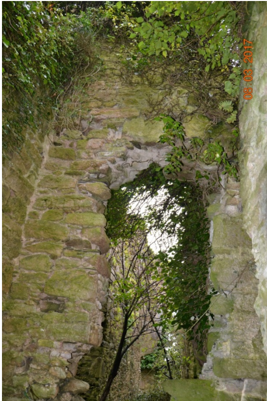
Photo 44 – Area 3. Lintel in poor repair.
