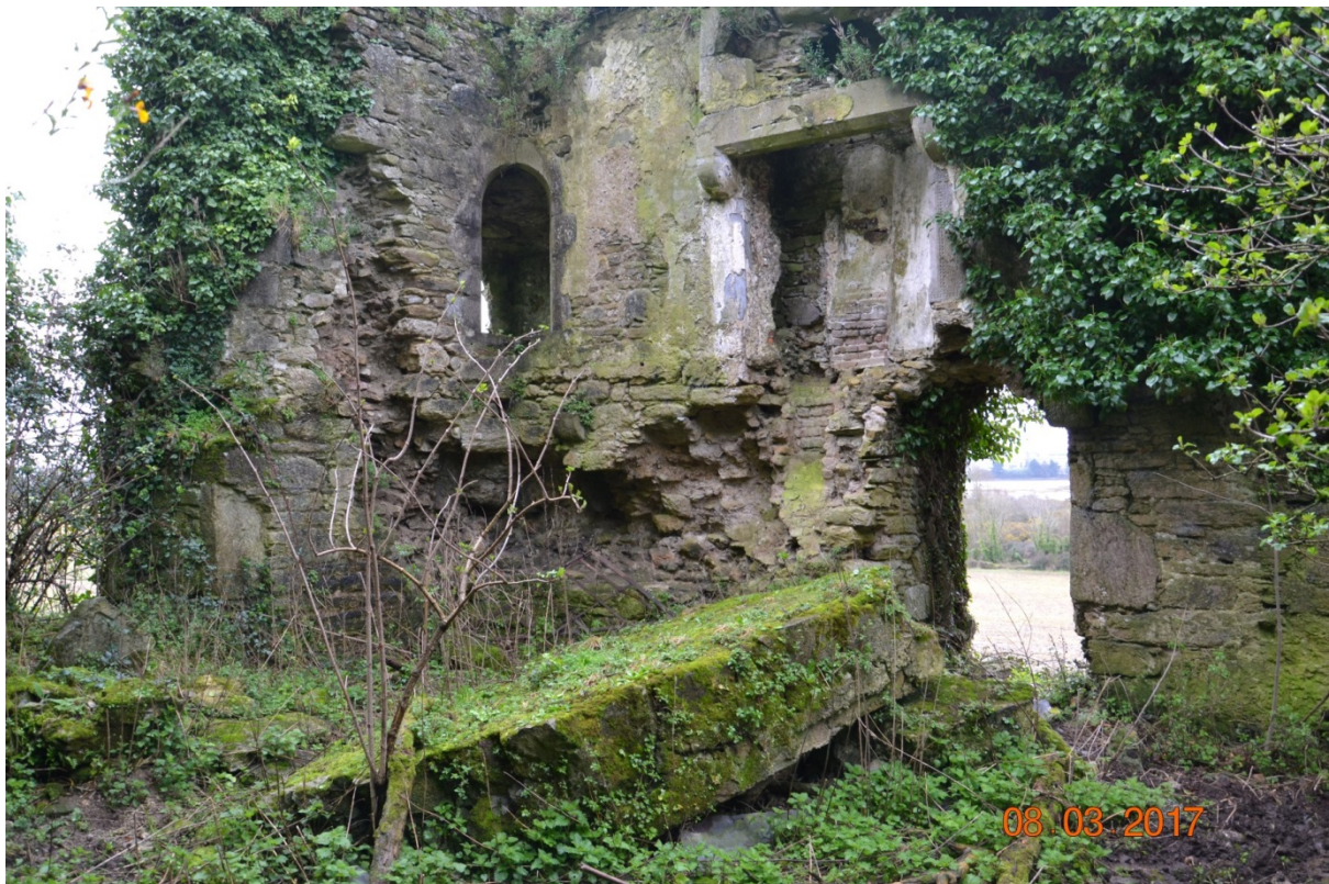
Photo 47 – Area 4. View of the bartizan / South Eastern corner of Castle Warren House. Note the significant loss of masonry / mortar. Also note the significant wall collapse in the foreground.
