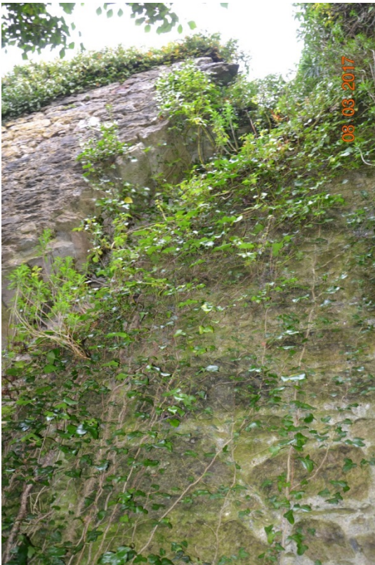
Photo 43 – Area 3. Chimney cuts up through the wall.
